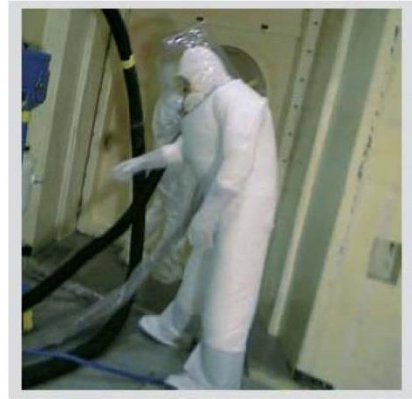
Fig: Operators wears full PPE with fresh air supply for working in contaminated area
