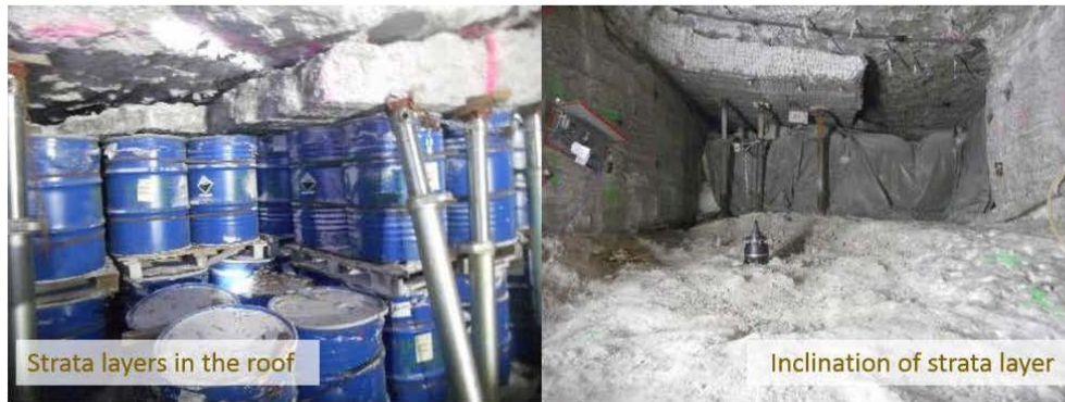
Figure 4: damaged roof and inclination of strata layer
