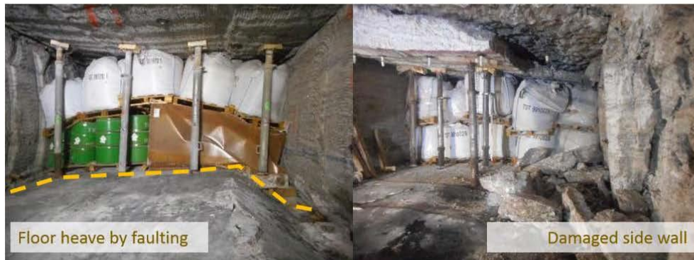
Figure 5: Floor heave and damaged side wall
